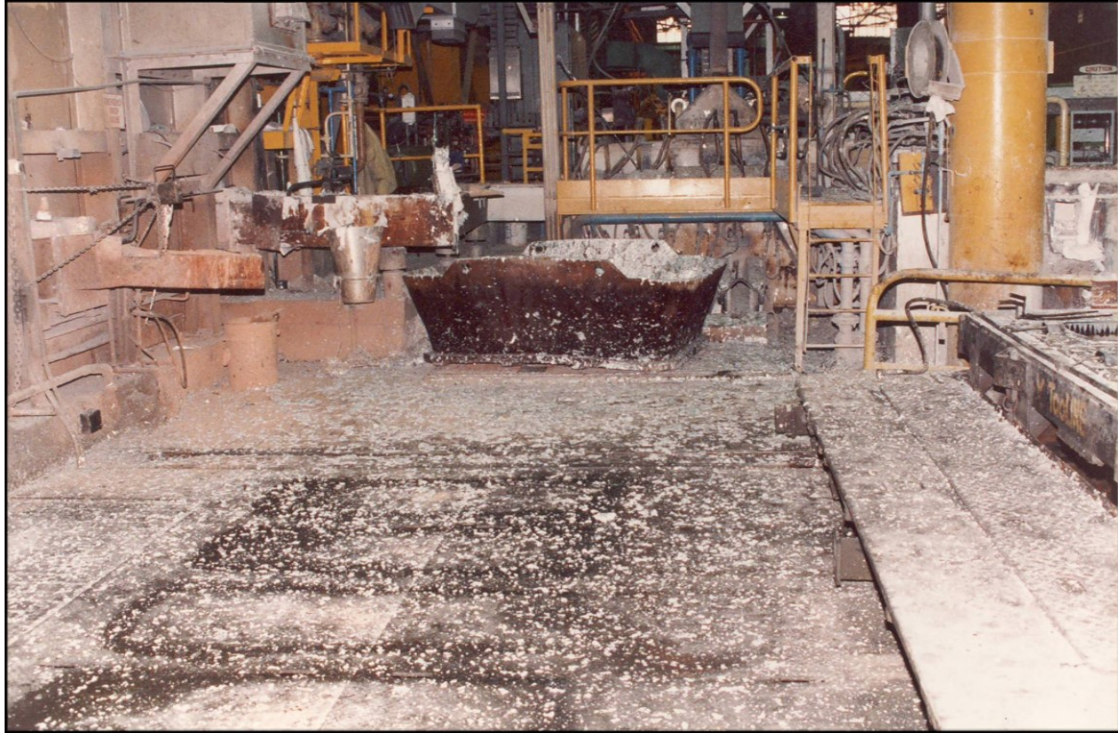
Figure 1. Common physical reaction explosion involving a drain pan.
